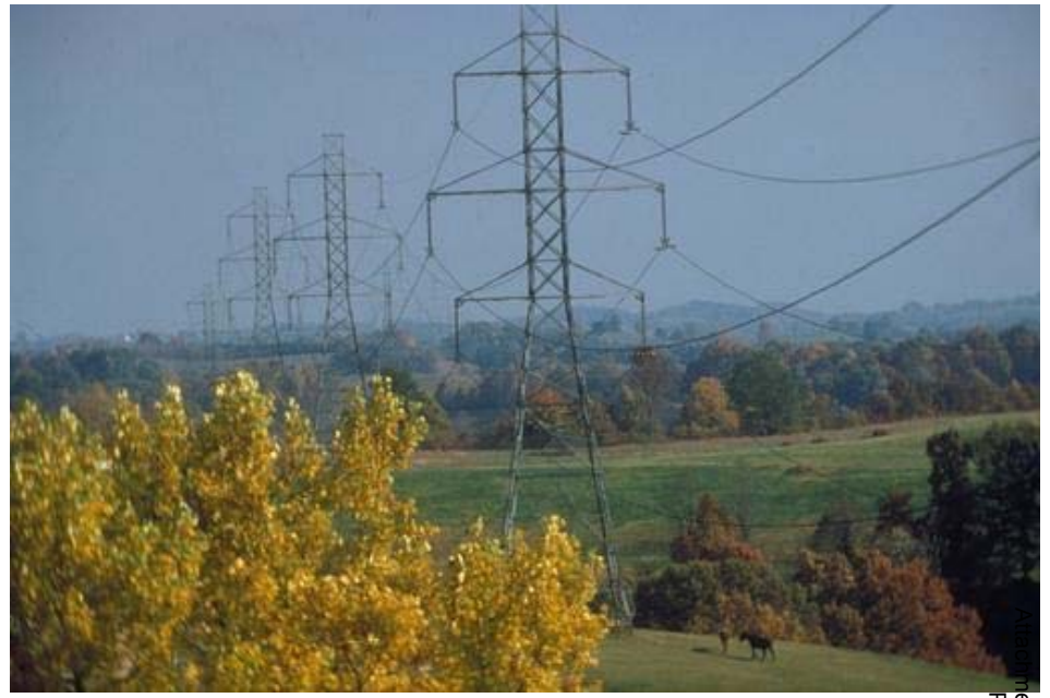
345-kV Transmission Line
