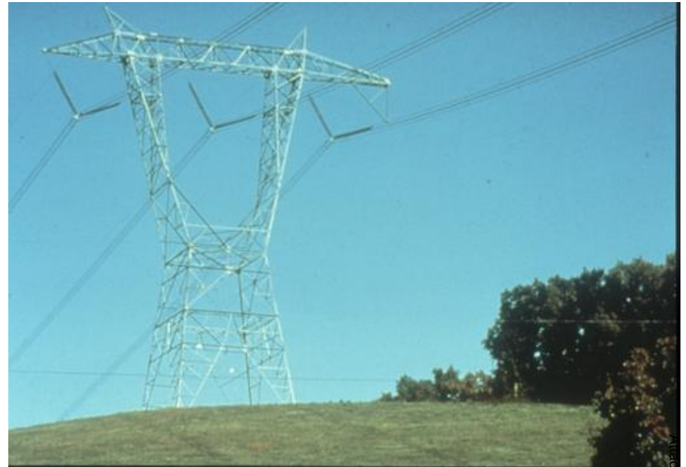
765-kV Transmission Line
