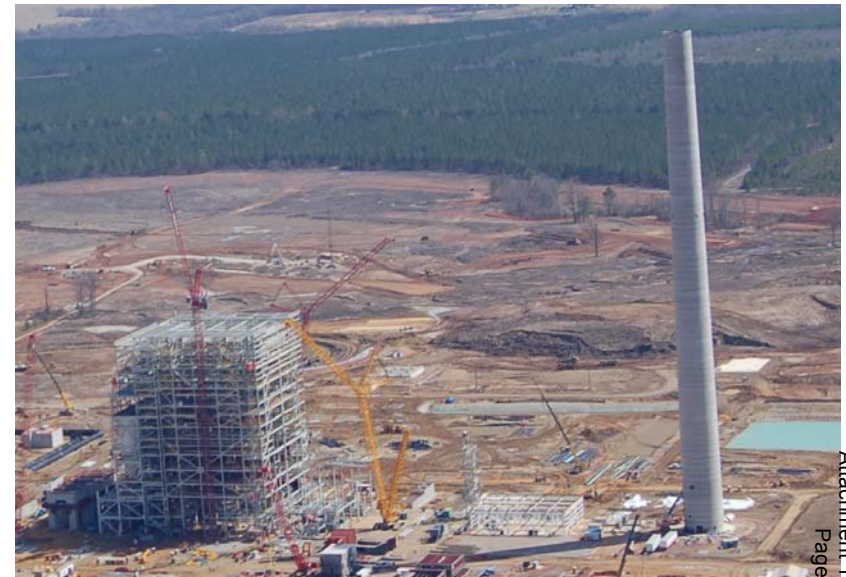
John W. Turk Jr. Ultra-Supercritical Coal Plant
