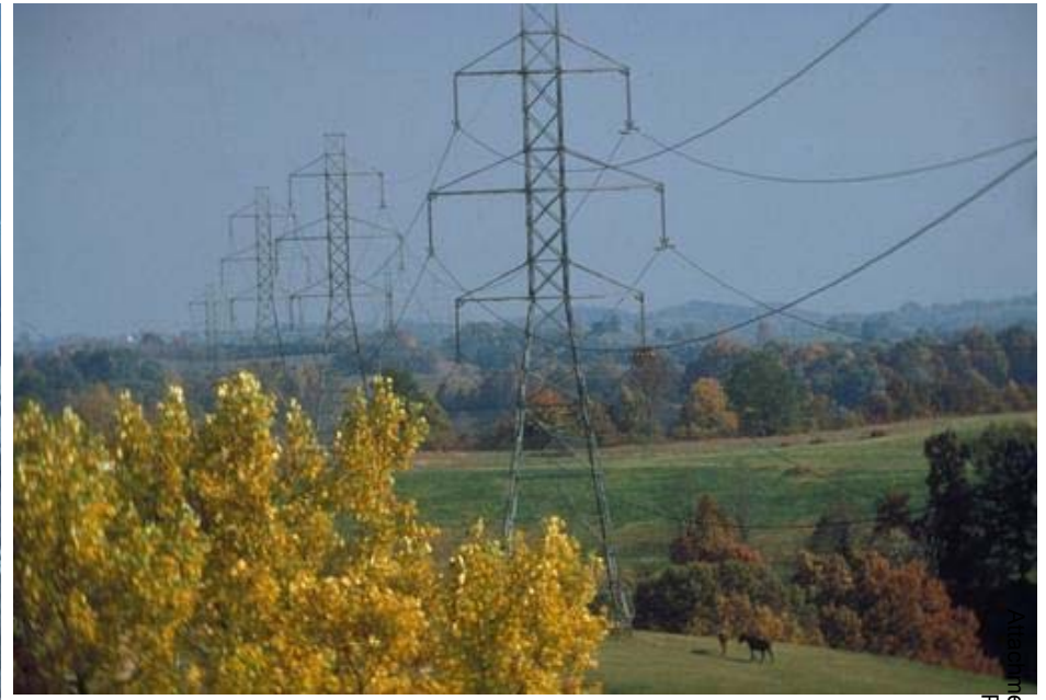
345-kV Transmission Line
