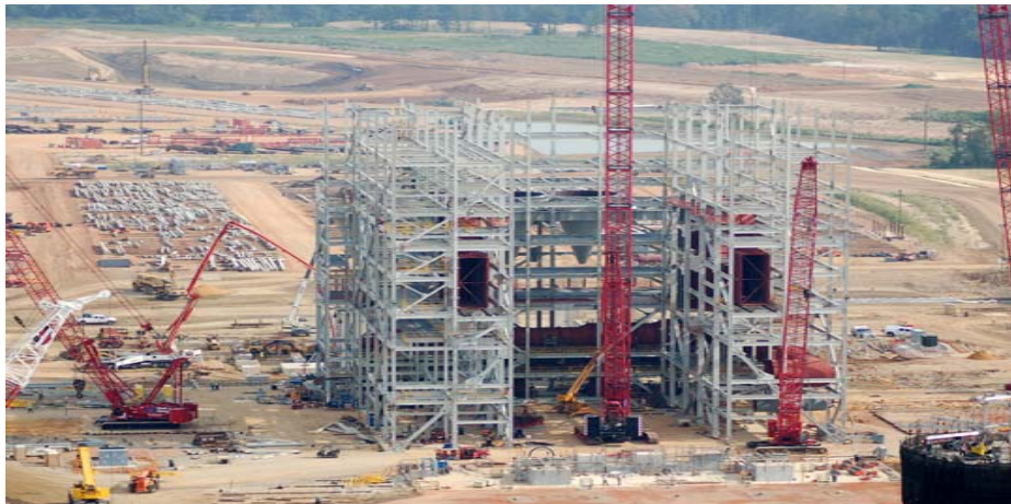
John W. Turk Jr. Ultra-Supercritical Coal Plant
