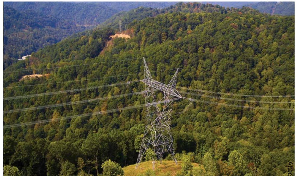
765-kV Transmission Line – Wyoming-Jacksons Ferry (WV)
