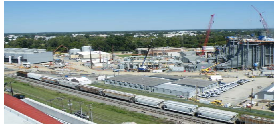
J. Lamar Stall Combined-Cycle Gas Plant
