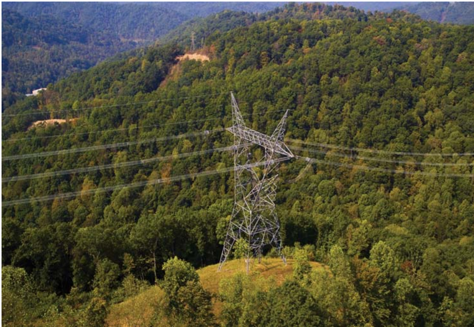
765-kV Transmission Line (Wyoming-Jacksons Ferry)
