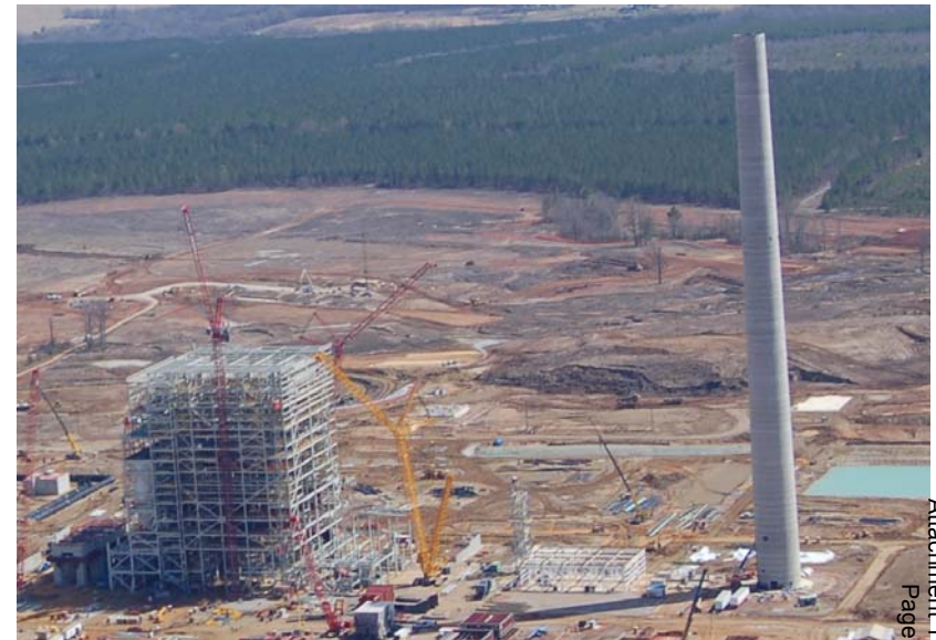
John W. Turk Jr. Ultra-Supercritical Coal Plant
