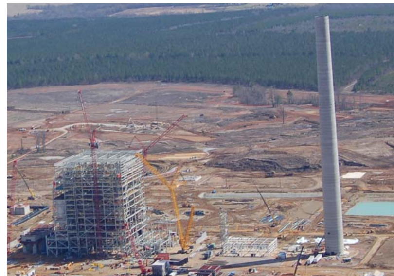
John W. Turk Jr. Ultra-Supercritical Coal Plant
