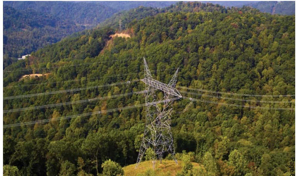
765-kV Transmission Line – Wyoming-Jacksons Ferry (WV)
