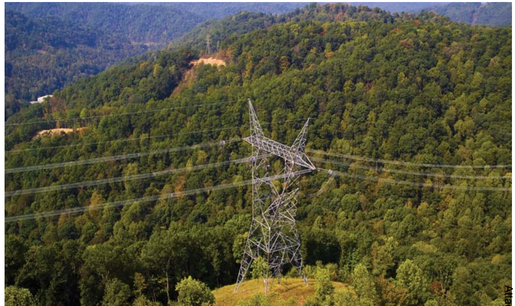
765-kV Transmission Line – Wyoming-Jacksons Ferry (WV)
