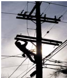
One of the largest U.S. electricity distributors
