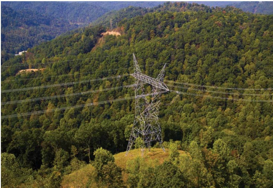
765-kV Transmission Line (Wyoming-Jacksons Ferry)
