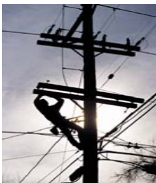
One of the largest U.S. electricity distributors
