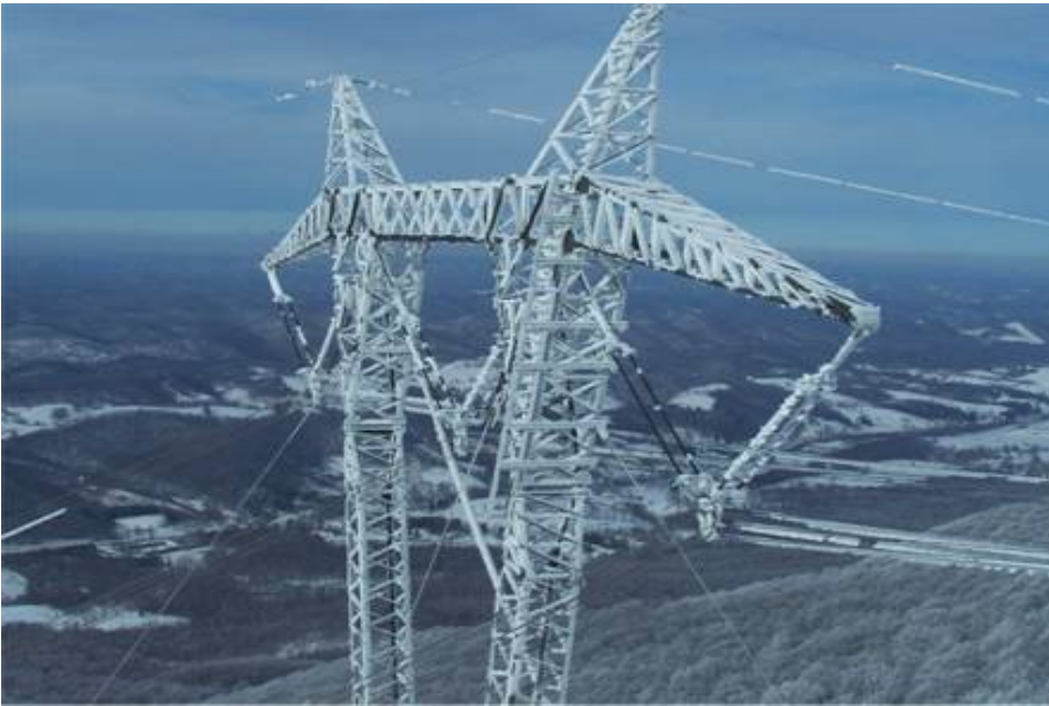
765-kV Transmission Line
