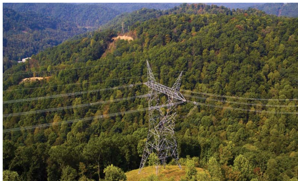
765-kV Transmission Line – Wyoming-Jacksons Ferry (WV)
