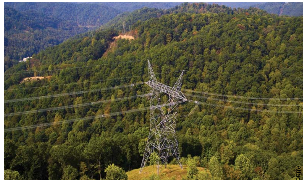
765-kV Transmission Line – Wyoming-Jacksons Ferry (WV)
