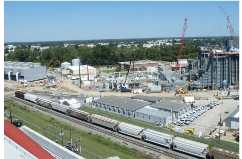
J. Lamar Stall Combined-Cycle Gas Plant
