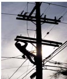
One of the largest U.S. electricity distributors
