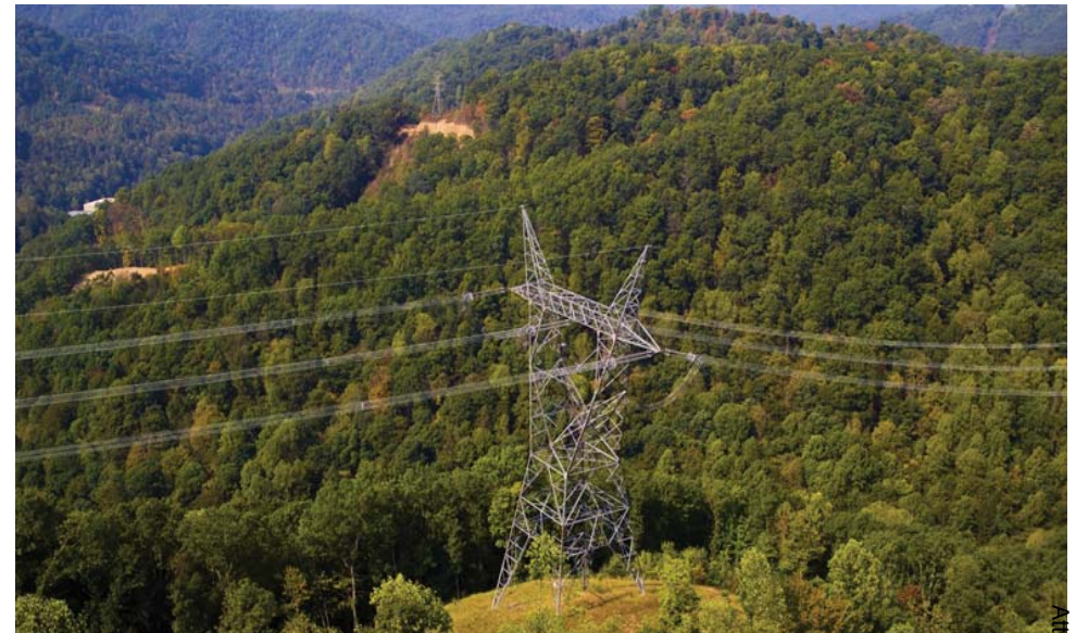
765-kV Transmission Line – Wyoming-Jacksons Ferry (WV)
