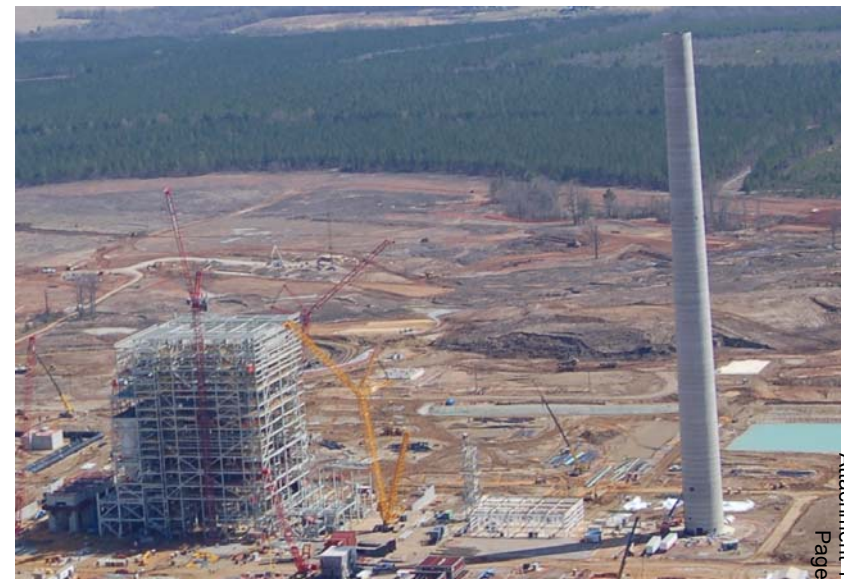
John W. Turk Jr. Ultra-Supercritical Coal Plant
