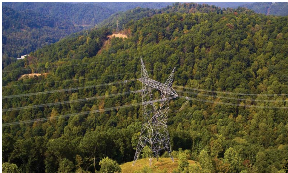
765-kV Transmission Line – Wyoming-Jacksons Ferry (WV)
