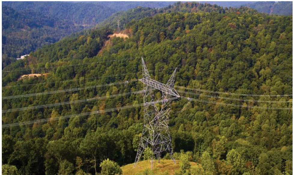
765-kV Transmission Line – Wyoming-Jacksons Ferry (WV)
