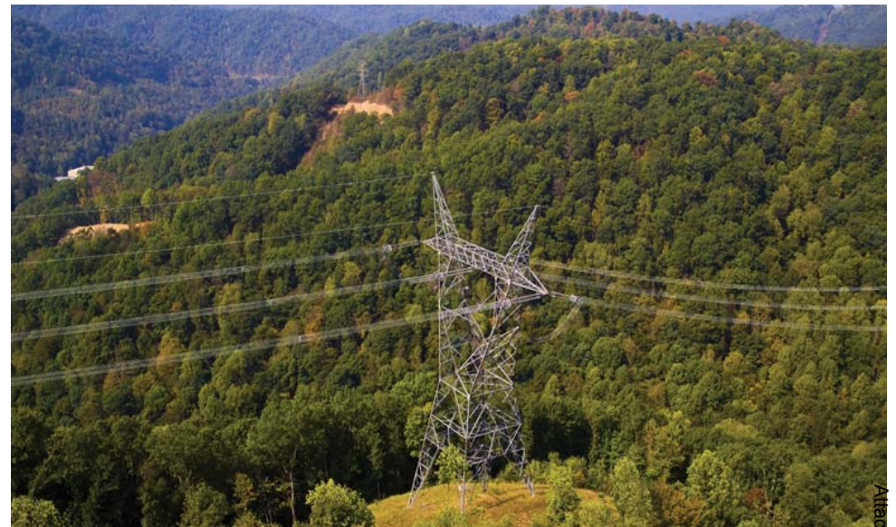
765-kV Transmission Line – Wyoming-Jacksons Ferry (WV)
