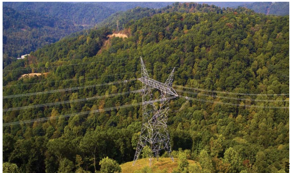
765-kV Transmission Line – Wyoming-Jacksons Ferry (WV)
