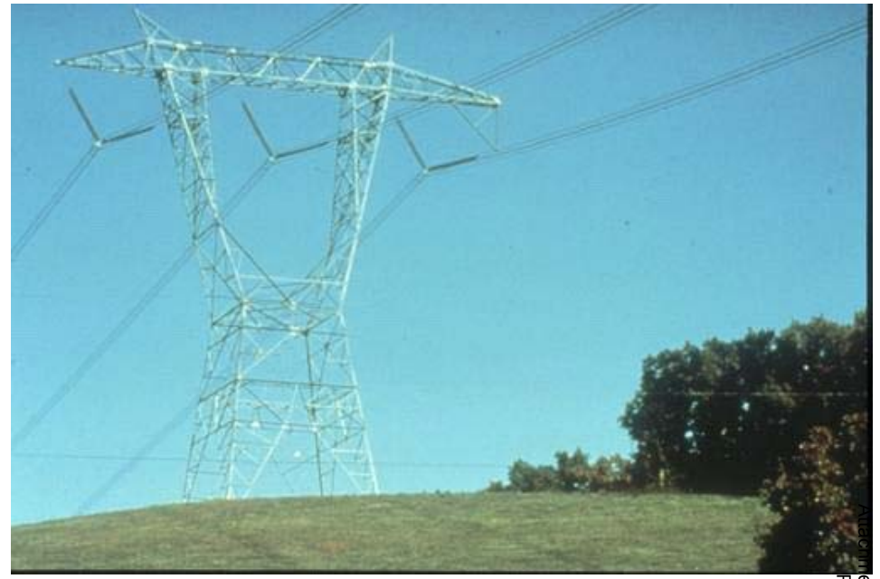
765-kV Transmission Line
