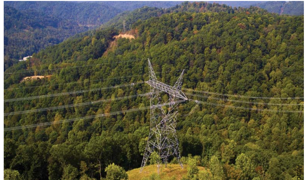
765-kV Transmission Line – Wyoming-Jacksons Ferry (WV)
