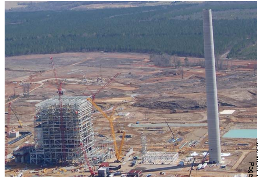
John W. Turk Jr. Ultra-Supercritical Coal Plant
