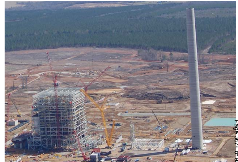
John W. Turk Jr. Ultra-Supercritical Coal Plant
