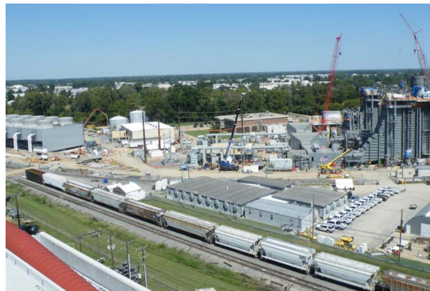
J. Lamar Stall Combined-Cycle Gas Plant
