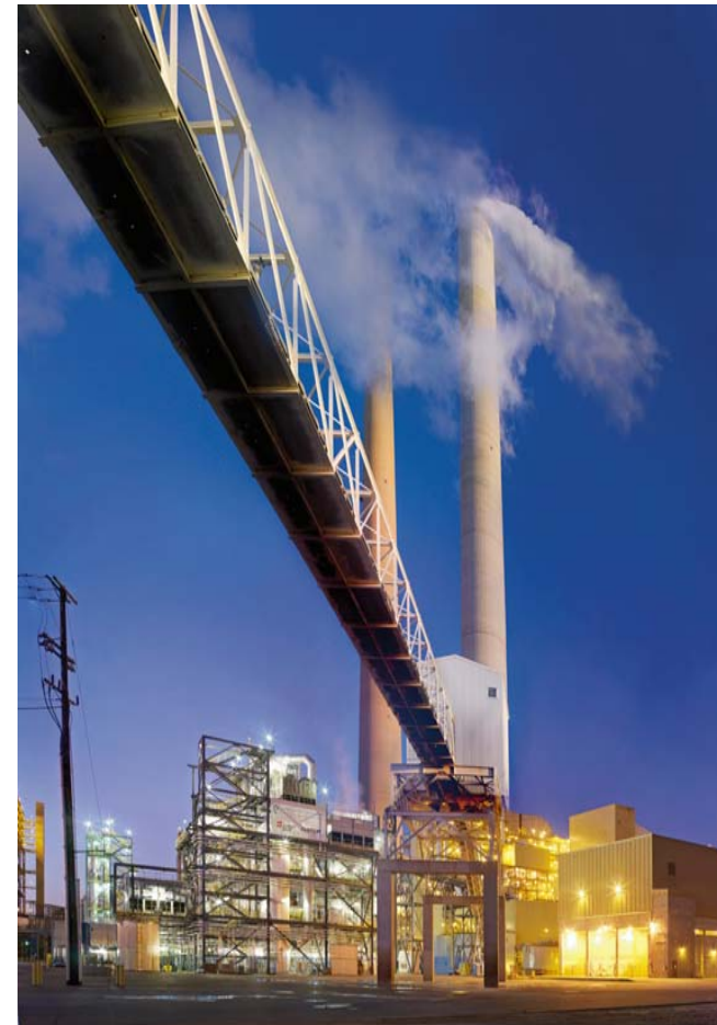
Carbon Capture and Storage project Mountaineer Plant - New Haven, WV
